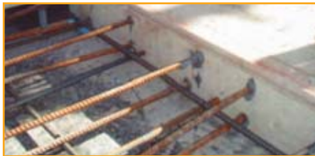
Starters bar anchored to slab prior to pour of adjoining floor slab, shallow depth and close to edge with A7 Injection.
